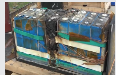
Figure 5: BESS Module (Our Next Energy, Inc.) Post-Thermal Runaway Test using GORE Battery Insulation
