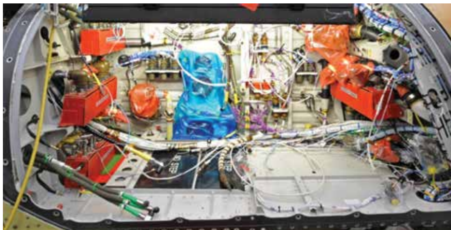
Figure 2: Typical Cable Installation in an Airframe
