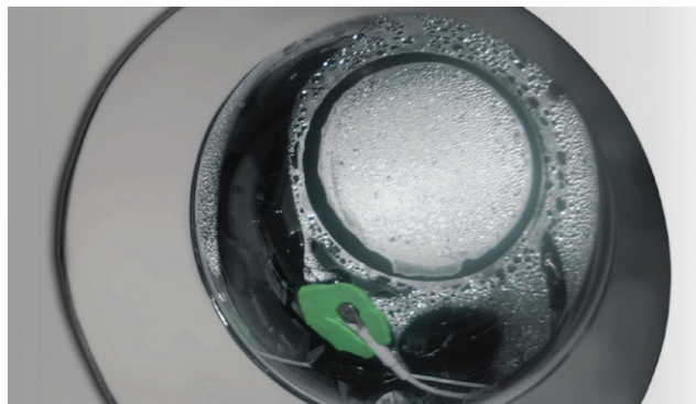
Figure 1: Desiccant could not prevent severe condensation from forming and becoming trapped within this sealed enclosure.
